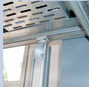
Vertical pipe connection solved using the outlet platet
